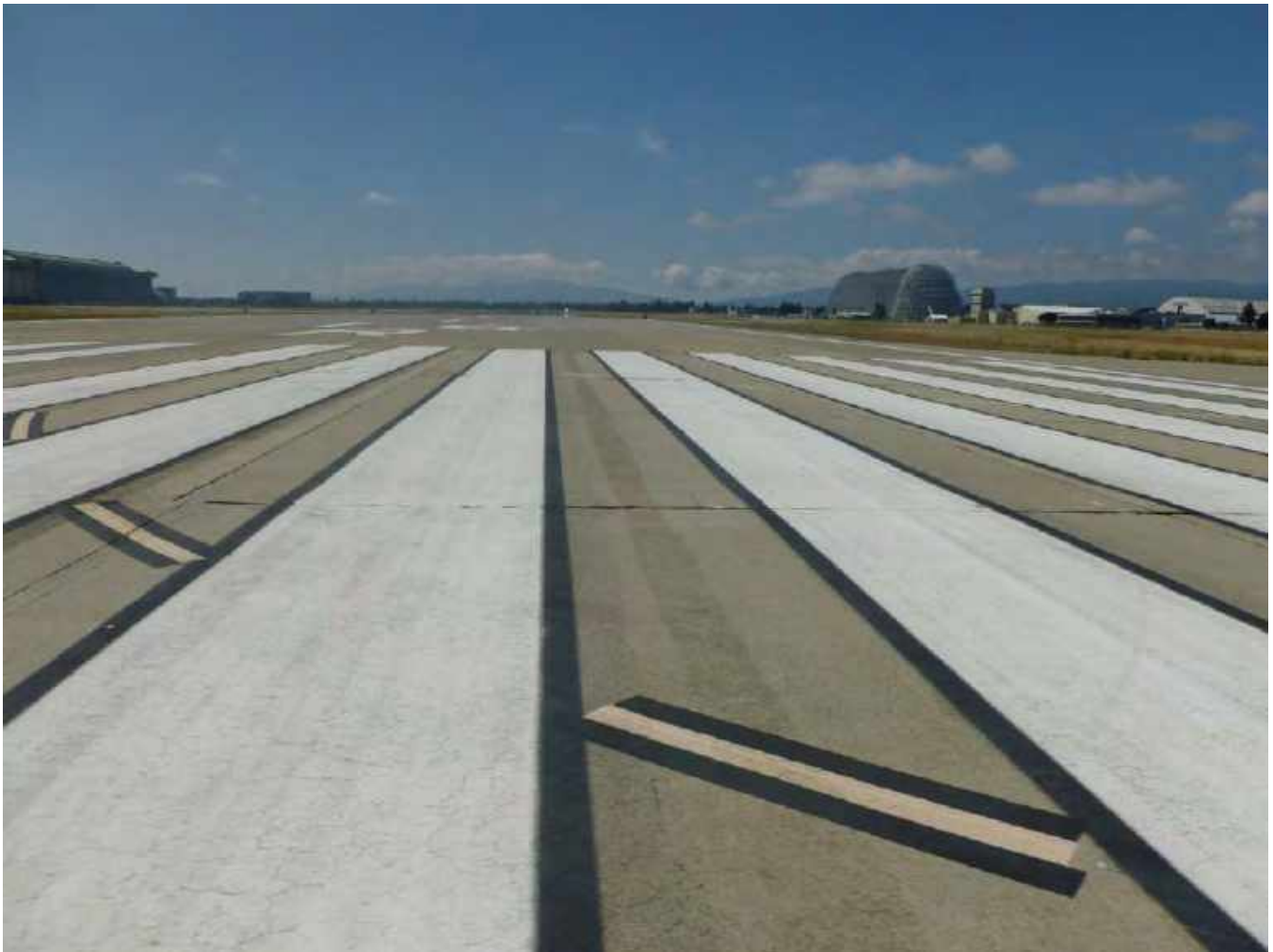
Detail view of Runway 14R-32L looking south (Source: AECOM 2013)
