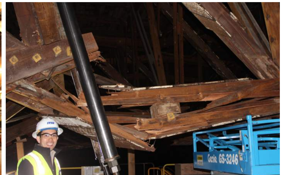
Damaged chord member viewed from access tower
