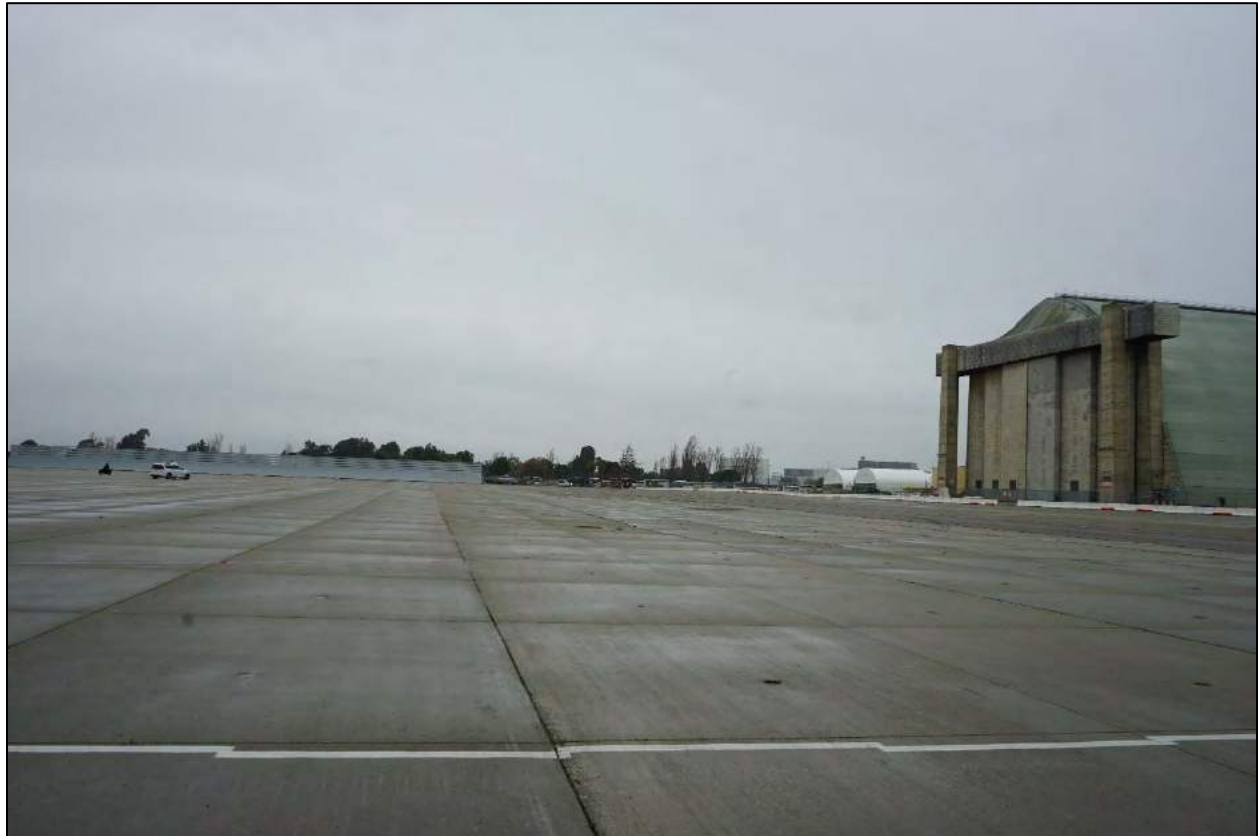
Photograph 6: North portion of East MF1002 exhibiting typical conditions; note Hangar 3 north façade at right.
