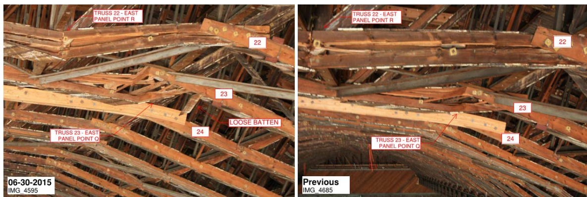
Figure 1. Truss damage progression at Trusses 22 and 23 East near Panel Points R and Q.
