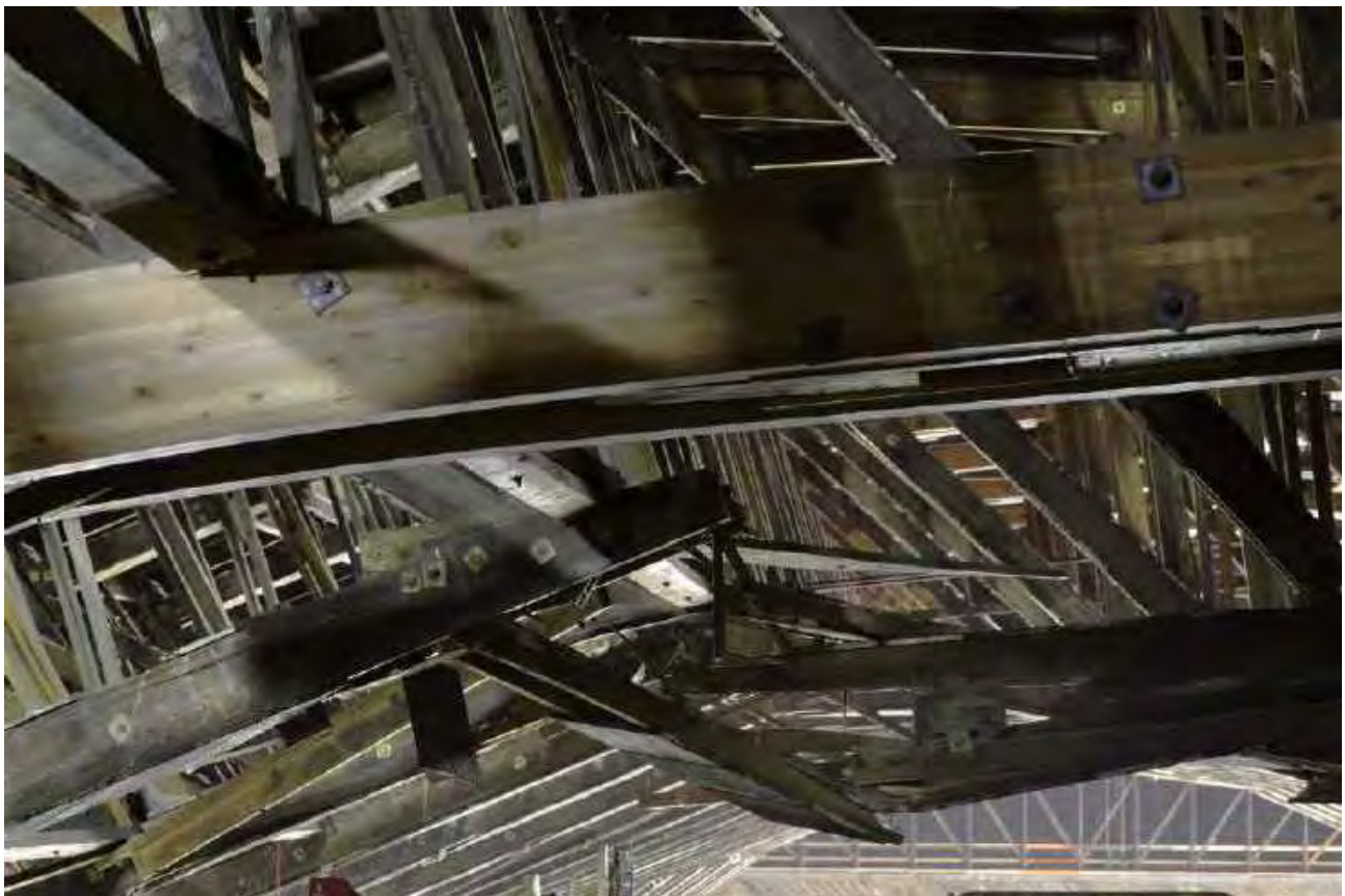
Figure 6. Broken bottom chord near top of truss.
