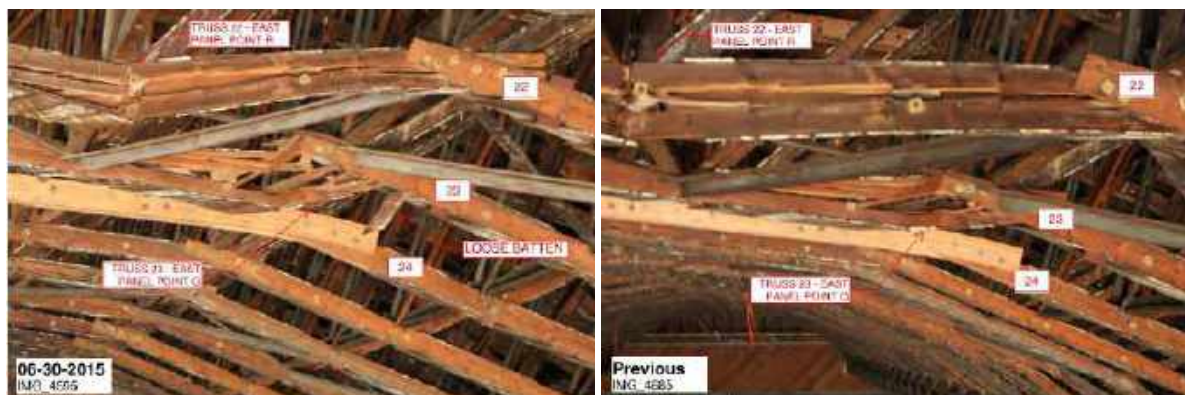
Figure 1. Truss damage progression at Trusses 22 and 23 East near Panel Points R and O.
