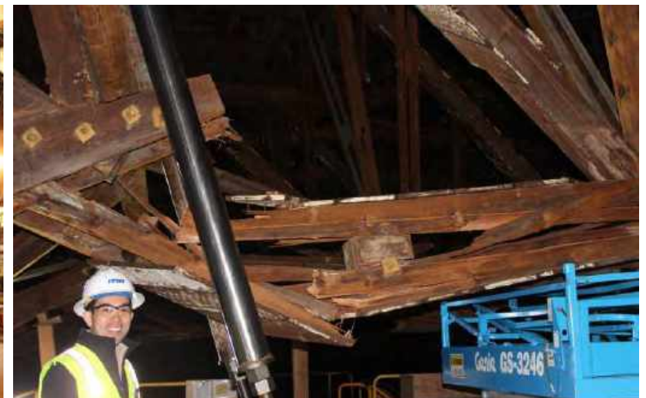
Damaged chord member viewed from access tower
